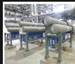
#904301.063 CELLECO CLEANPAC 350 CLEANING BANK SYSTEM
