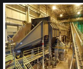
#109202.002 KONE VALMET DEBARKING SYSTEM 500 BDST/D SECTION REBUILT 2012
