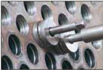
Expanded pipes with expansion grooving.
