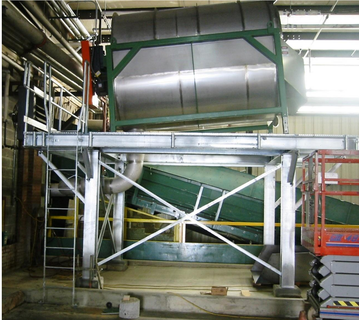
MTR Drum Screen Installed at Inland Empire - Spokane, WA
