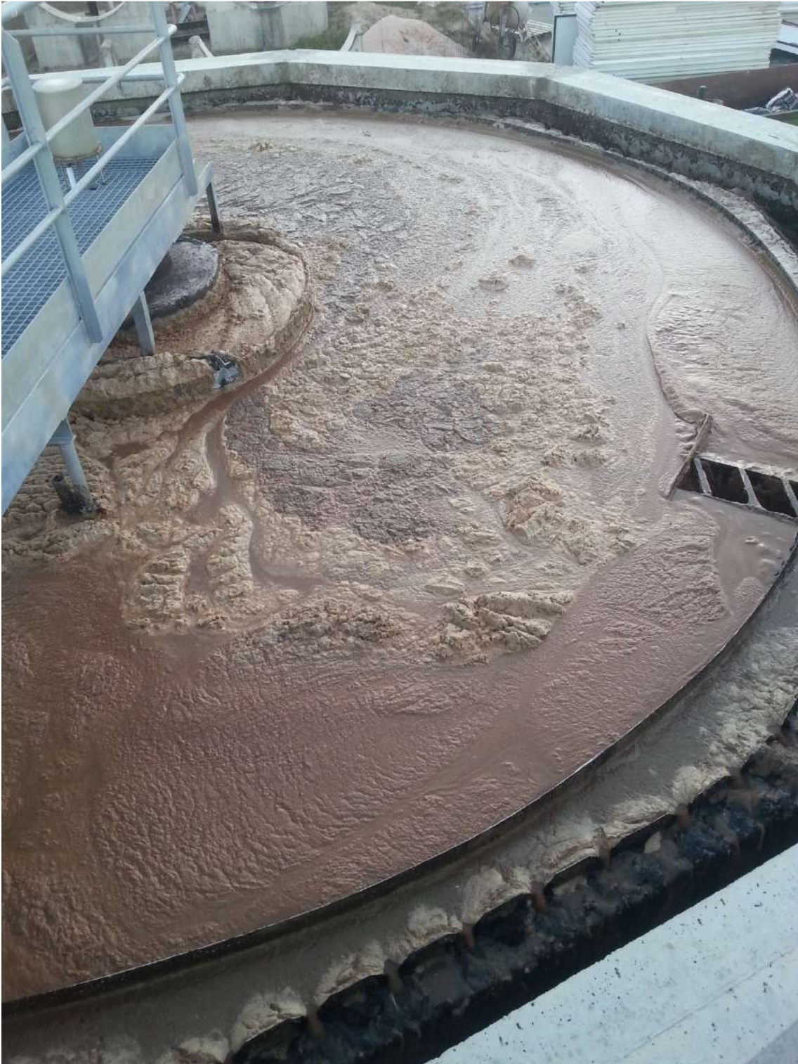
Picture 7 : Final Thickener with a bad quality of the flow due haven't made correctly the last commented stages and process.
