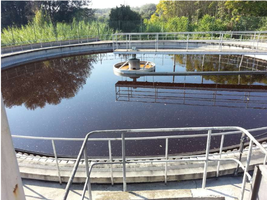
Picture 9 : Final settlement tank without floatin solids and wit a extreme good quality to pour the depurated wáter even directly to the river.
